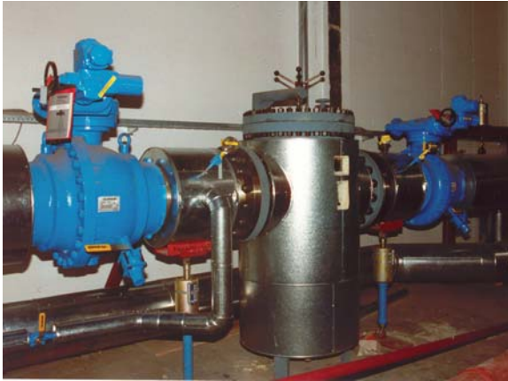
KHI ball valves in district heating system
