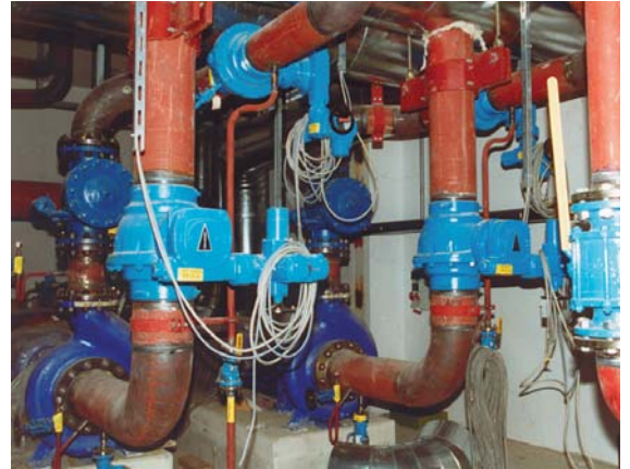
KHI ball valves in district heating system
